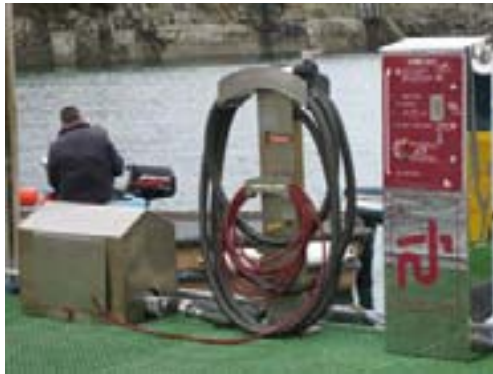
Sewage pump-out facility at Berrills Yard Pontoon
